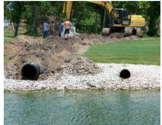
Figure 1, drain line/@ 18 fairway
