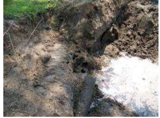
Fig. 4, Existing 15" & 6" drains discovery on lot #315.
